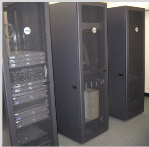
The Telfair County Schools datacenter, with the 2X ApplicationServer and 2X ThinClientServer installed.
